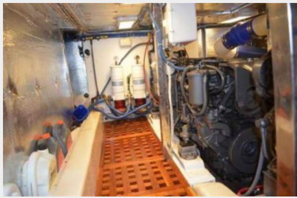
Main Engine Room with Yanmar Main Engine.
