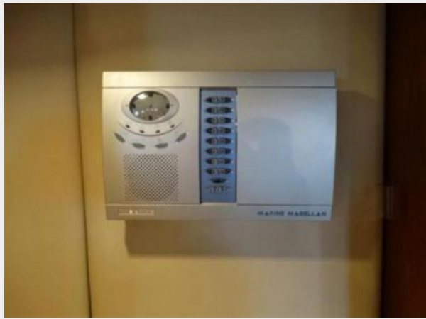
Security system panel
