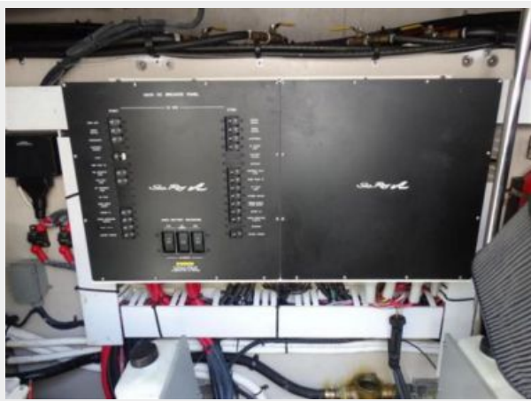
Engine rm breaker panel
