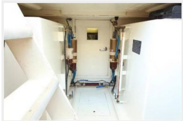
Fuel Tanks with filters and sight glass
