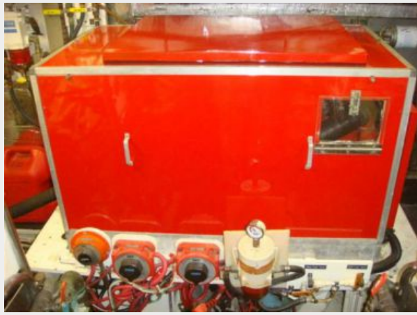
52' Cheoy Lee generator sound box
