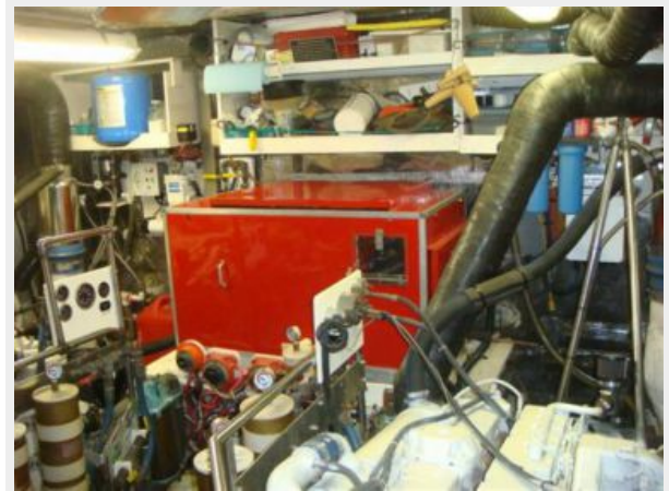
52' Cheoy Lee engine room aft
