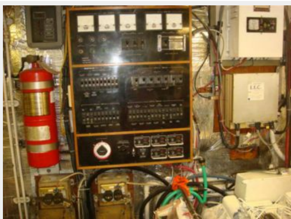
52' Cheoy Lee engine room forward
