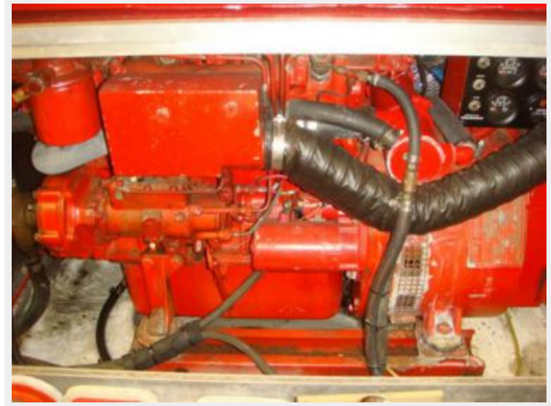
52' Cheoy Lee generator
