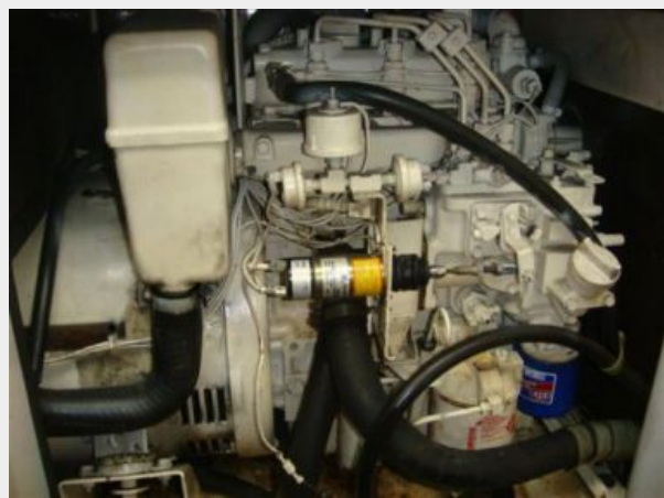
57' DeFever port generator
