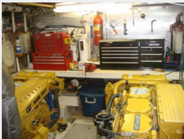
57' DeFever engine room forward
