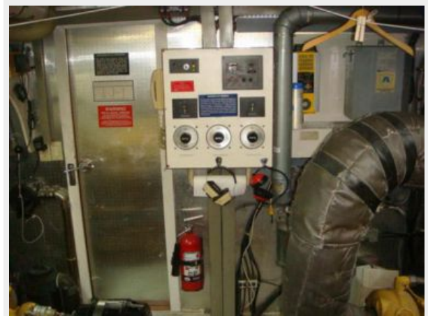
57' DeFever engine room aft
