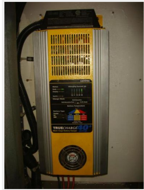
57' DeFever battery charger
