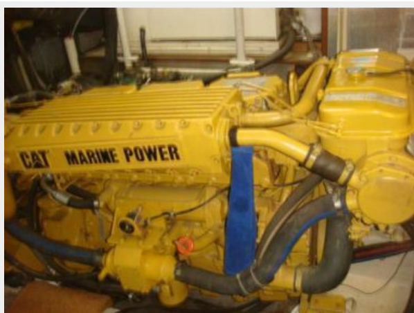
57' DeFever port main engine
