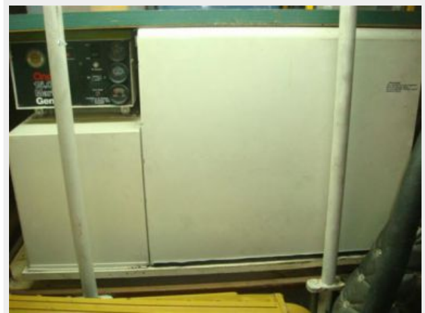
57' DeFever starboard generator sound box
