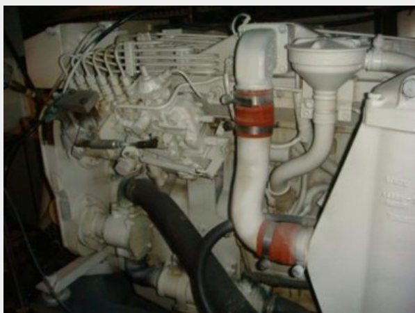
44' Carver starboard main engine photo2
