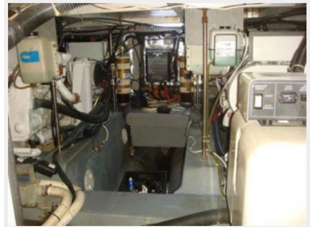
44' Carver engine room aft
