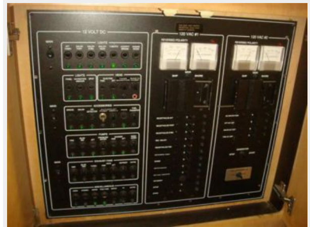
44' Carver electrical panel
