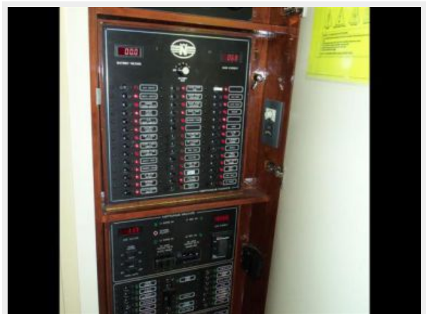
Companionway Electrical Panel
