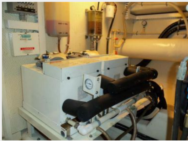
Chilled Water AC
