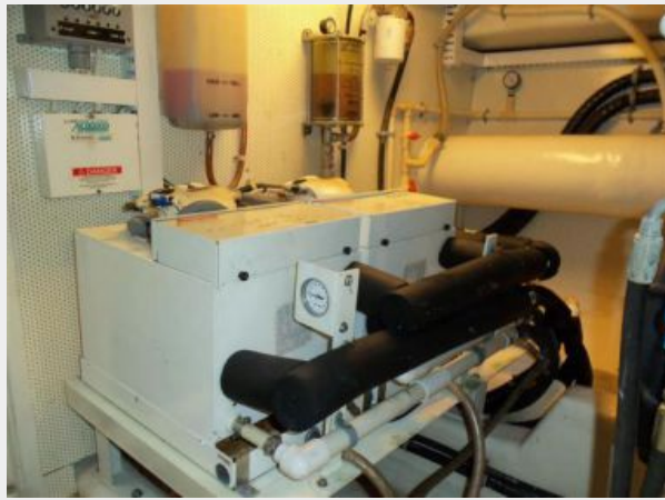
Chilled Water AC
