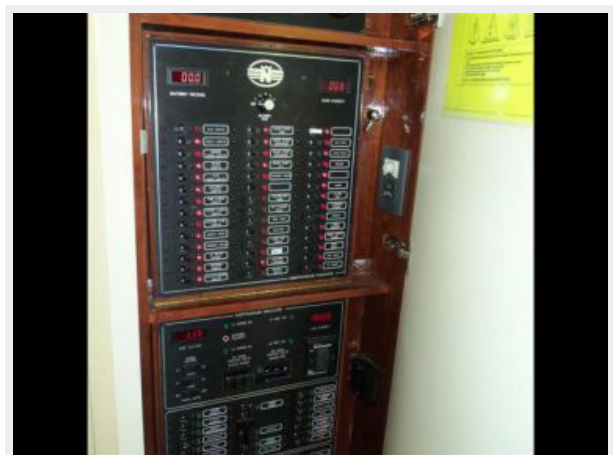
Companionway Electrical Panel
