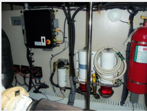
Engine Room Forward
