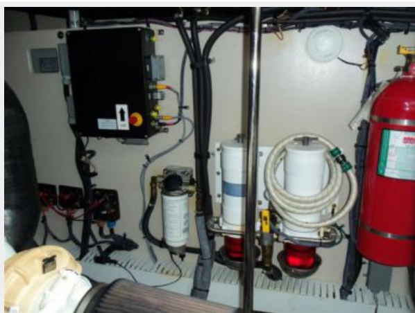
Engine Room Forward
