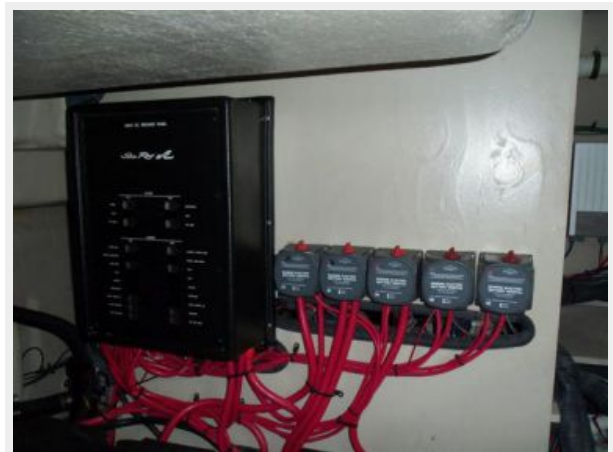
Electric Battery Switch
