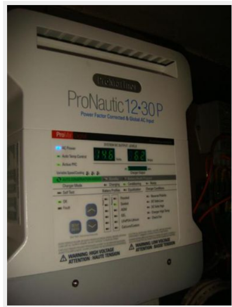
42' Catalina battery charger
