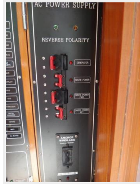
43' Selene electrical panel
