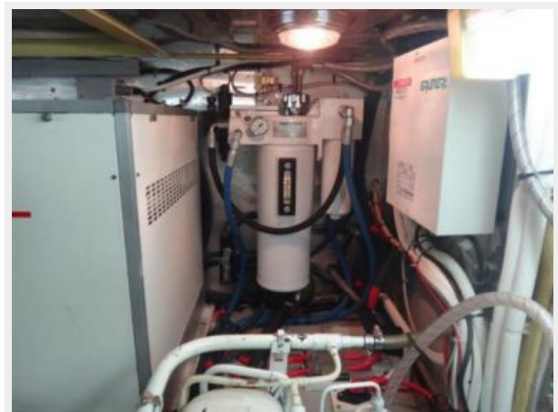
43' Selene engine room
