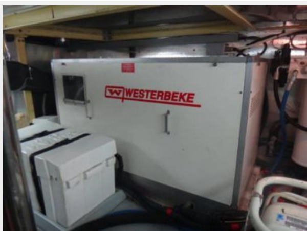
43' Selene Westerbeke Generator
