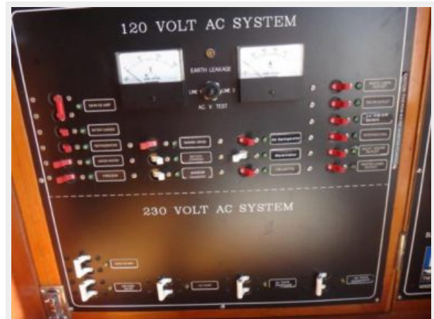
43' Selene electrical panel
