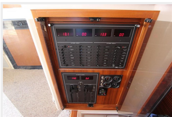
AC/DC Electrical Panel
