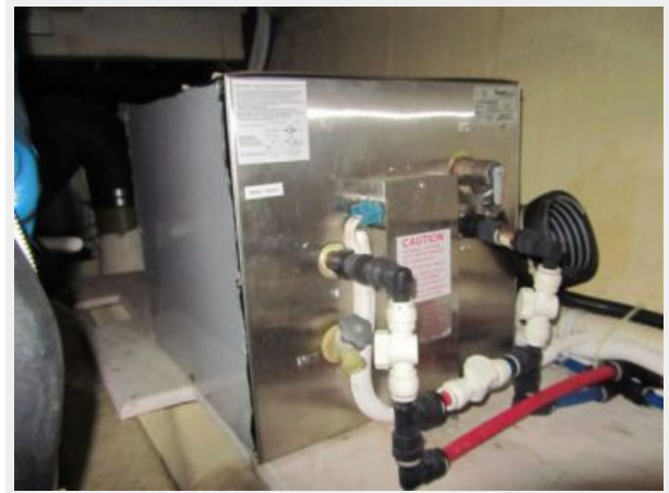
38' Carver water heater
