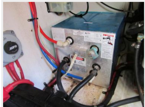
28' Cruisers water heater
