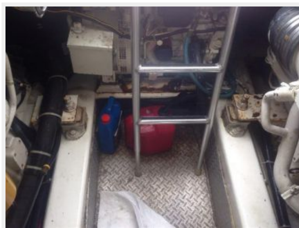
Generator in engine room
