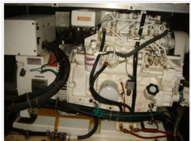
45' Ocean Alexander generator
