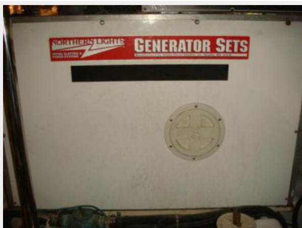
45' Ocean Alexander generator sound box
