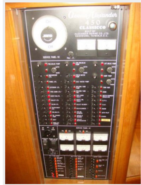
45' Ocean Alexander electrical panel
