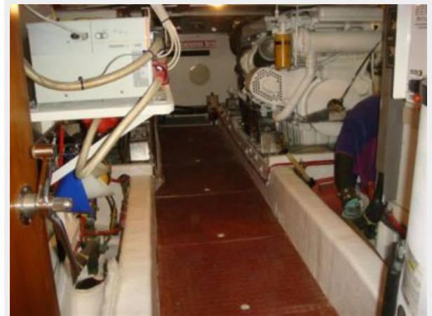
45' Ocean Alexander engine room aft
