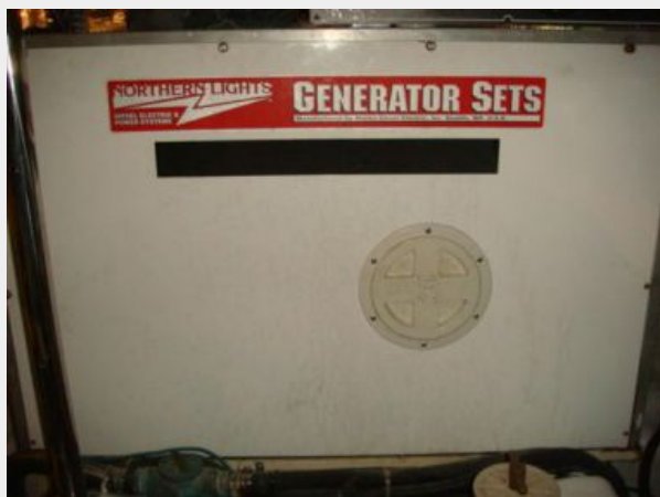
45' Ocean Alexander generator sound box
