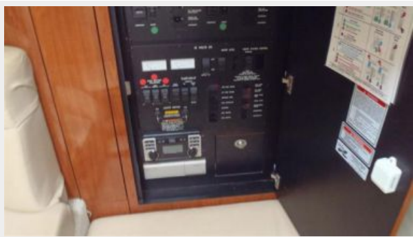
Main Power Panel
