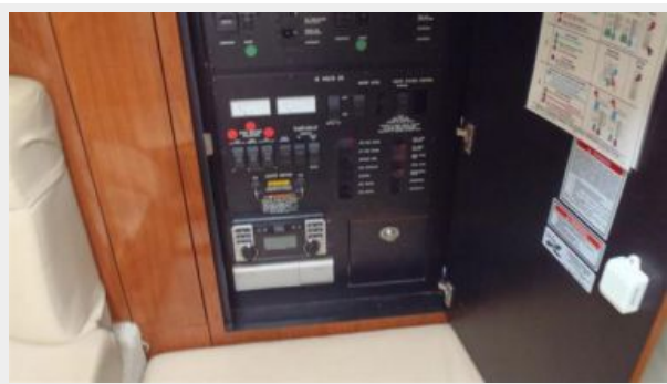
Main Power Panel
