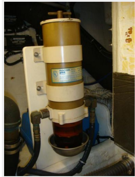
35' Tiara starboard Racor fuel filter
