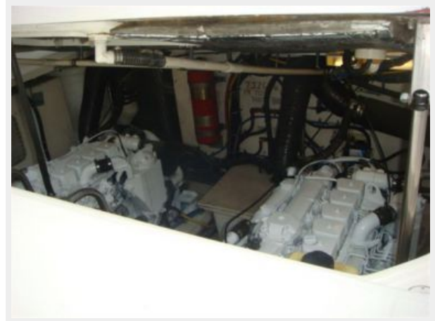
35' Tiara engine room access1
