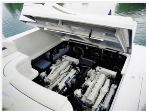
Engine Room access
