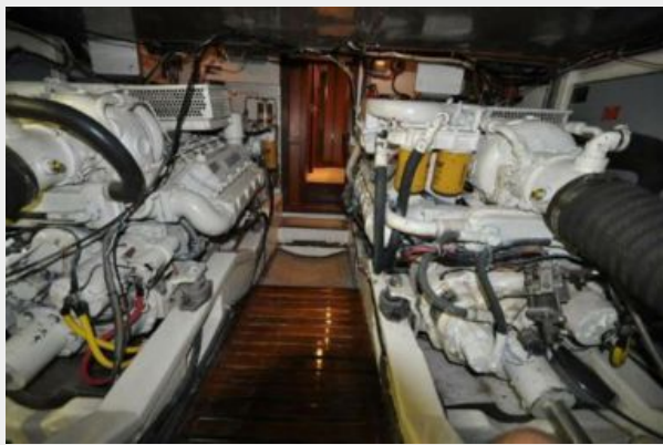
Engine room looking forward
