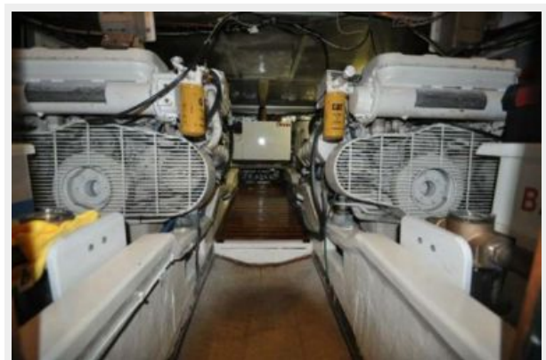
Engine room looking aft
