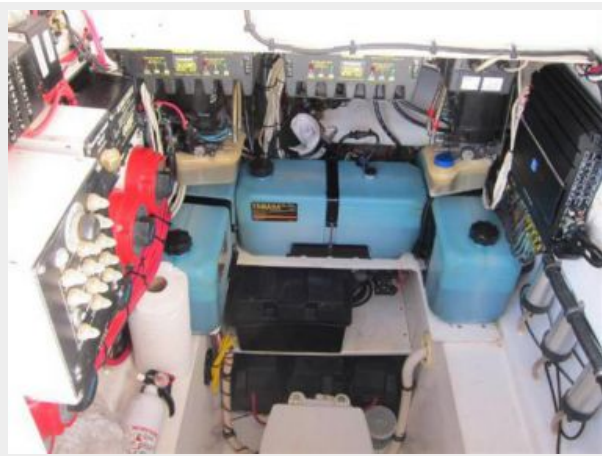
Oil tanks and batteries
