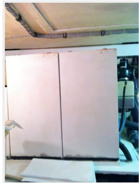
Engine Room Generator with Sound Shield
