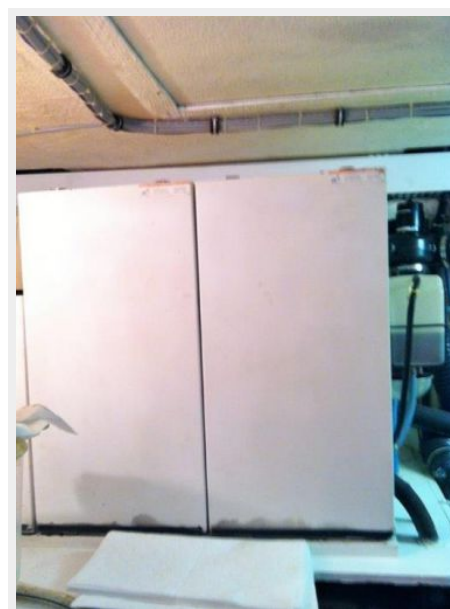
Engine Room Generator with Sound Shield
