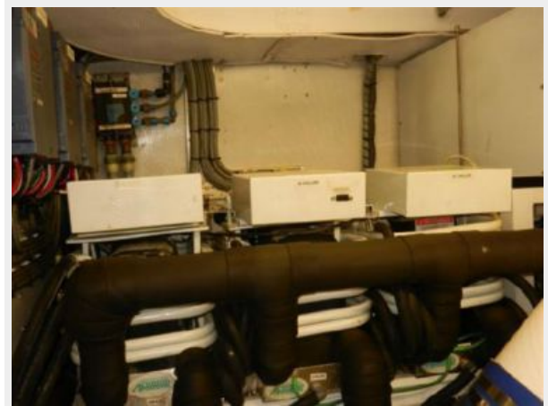
Aqua Air Chillers w/Frequency Drives
