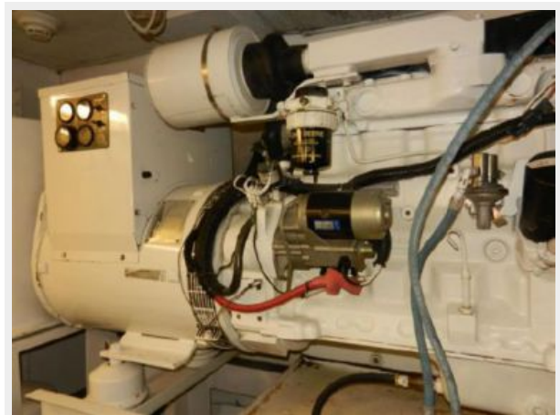
40 kw Northern Lights Generator
