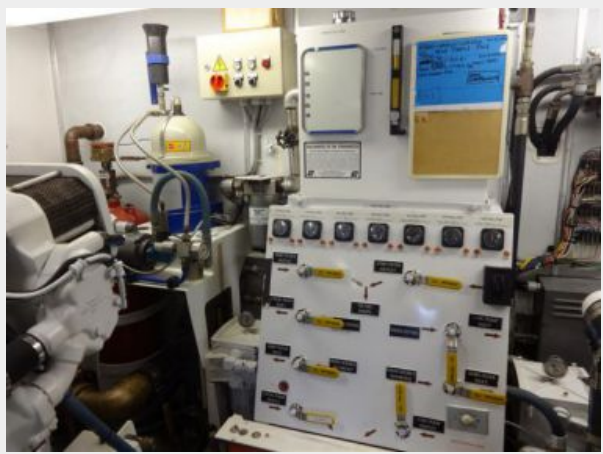
Fuel transfer manifold
