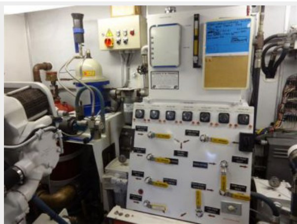
Fuel transfer manifold
