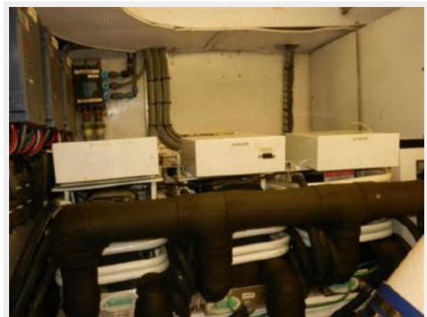
Aqua Air Chillers w/Frequency Drives
