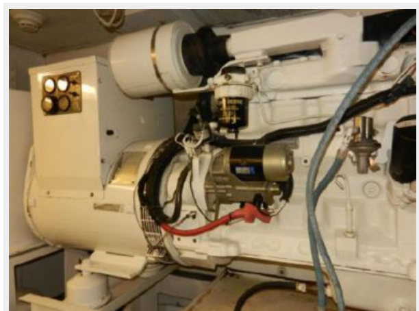
40 kw Northern Lights Generator
