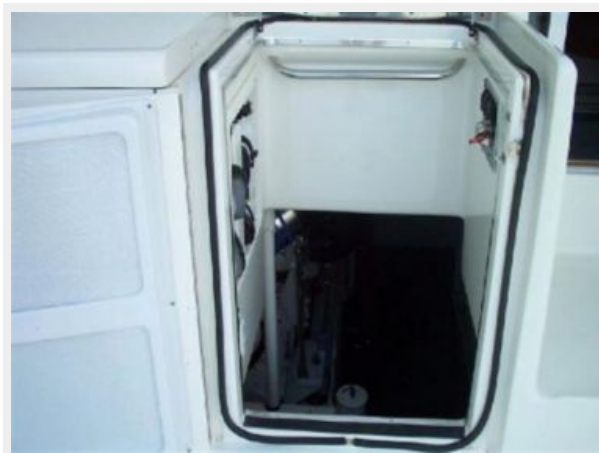
Engine Room Entrance
