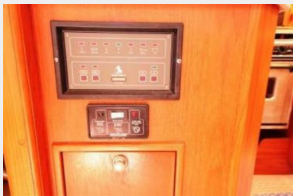
Island Packet 420 Generator Controls
