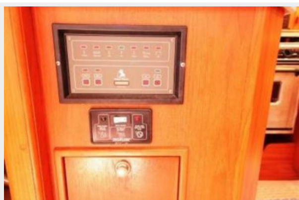
Island Packet 420 Generator Controls
