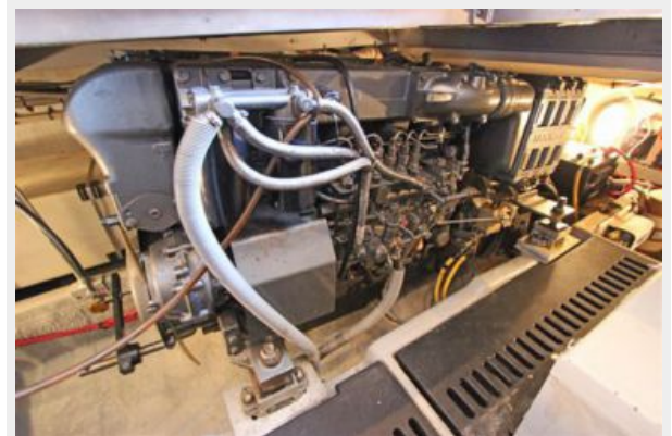
Starboard Yanmar Diesel Engine
