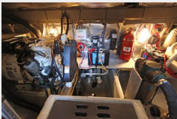
Engine Room Looking Forward
