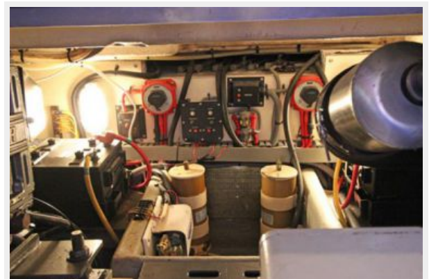
Engine Room Looking Aft
