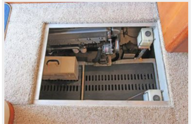
Salon Engine Room Access
