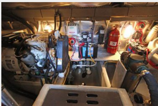
Engine Room Looking Forward
