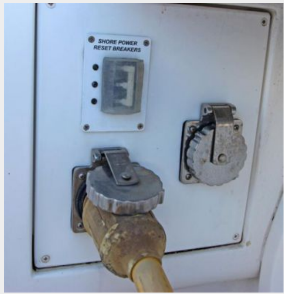
50 Amp Shore Power Service
