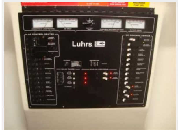
Electric panel ( in cabin)
