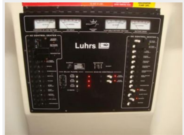
Electric panel ( in cabin)
