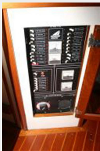
MAIN ELECTRIC PANEL
