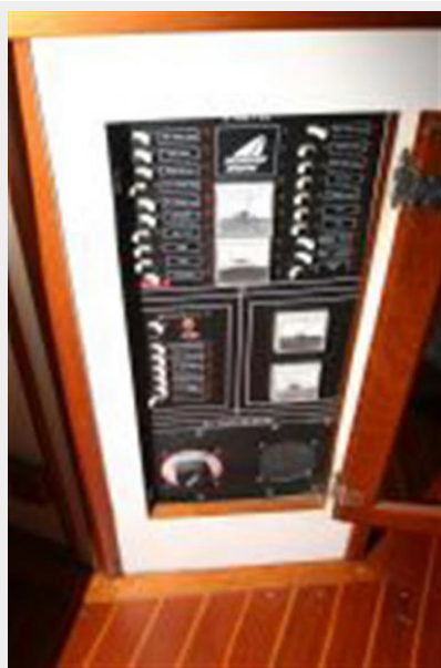
MAIN ELECTRIC PANEL
