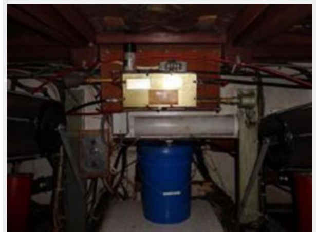
Aft Engine Room
