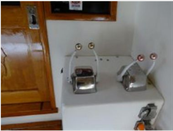
Lower Controls to Starboard
