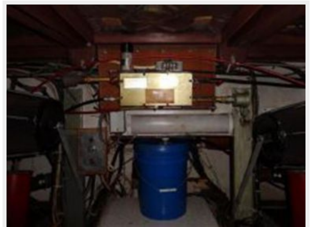
Aft Engine Room
