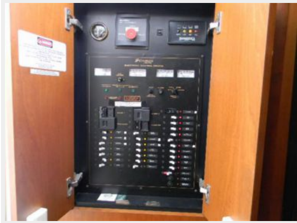
Main Distribution Panel
