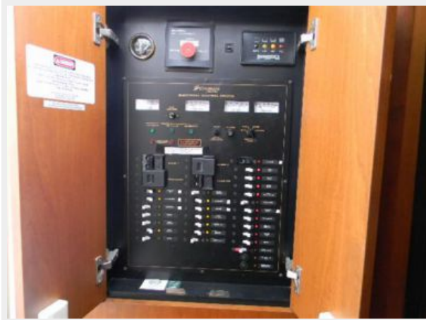
Main Distribution Panel
