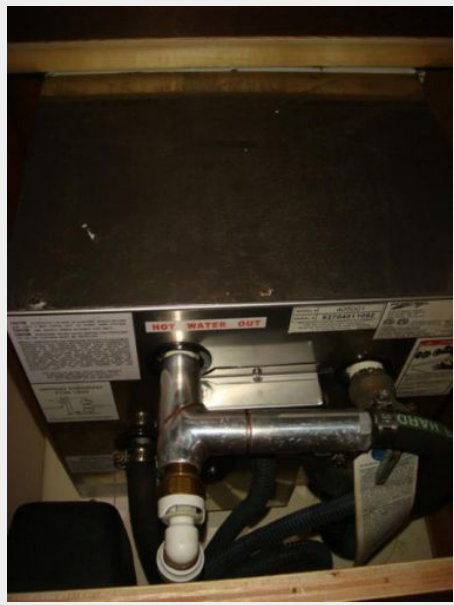
38' Hunter water heater
