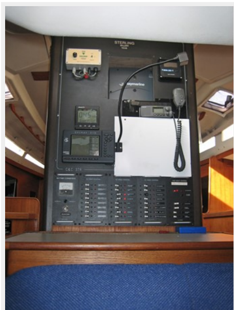
Electrical Panel/Nav Station
