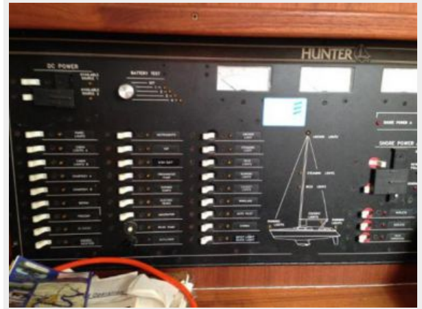
Electrical Breaker panel
