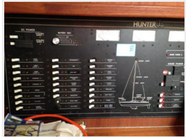
Electrical Breaker panel
