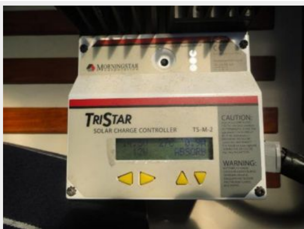
Solar Panel Control
