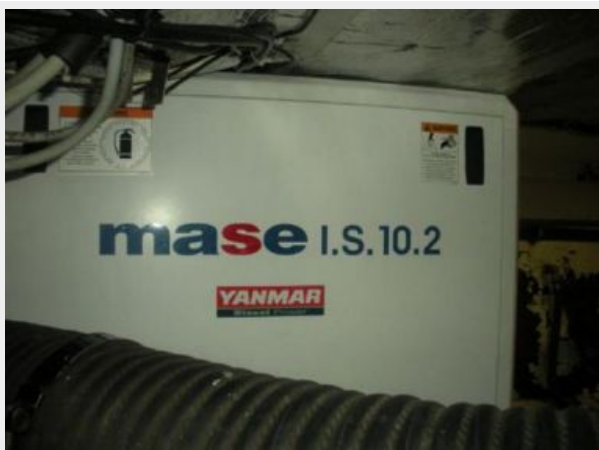
New Mase Generator - 10 Hours
