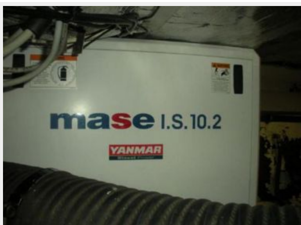
New Mase Generator - 10 Hours
