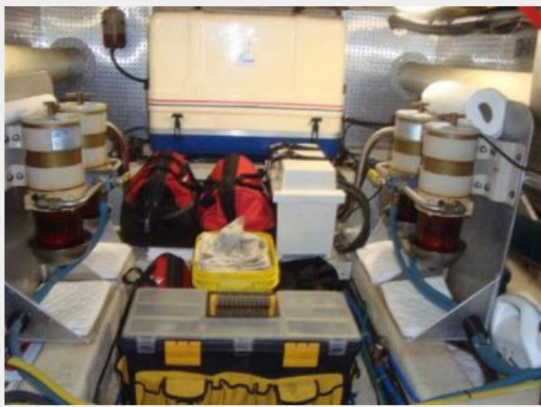
Generator in Sound Shield
