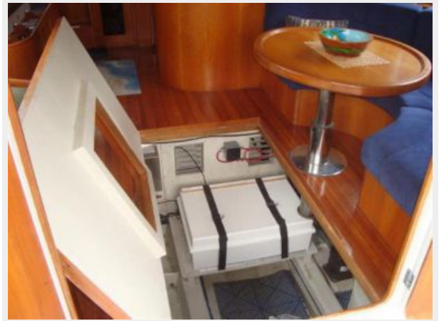
Open Hatch to batteries & storage - Salon
