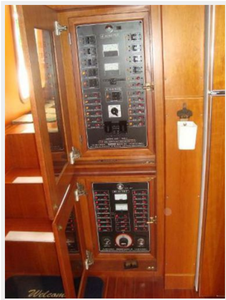
Main Electrical panels
